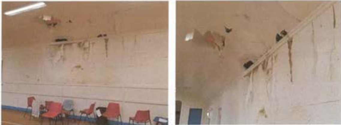
Main Hall - Ceiling and wall damage from water ingress through roof leak.
