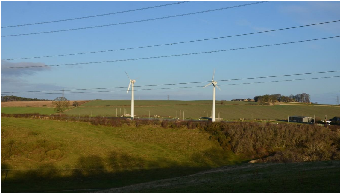
Figure 2.1: Domestic-scale wind turbines near Cousland
