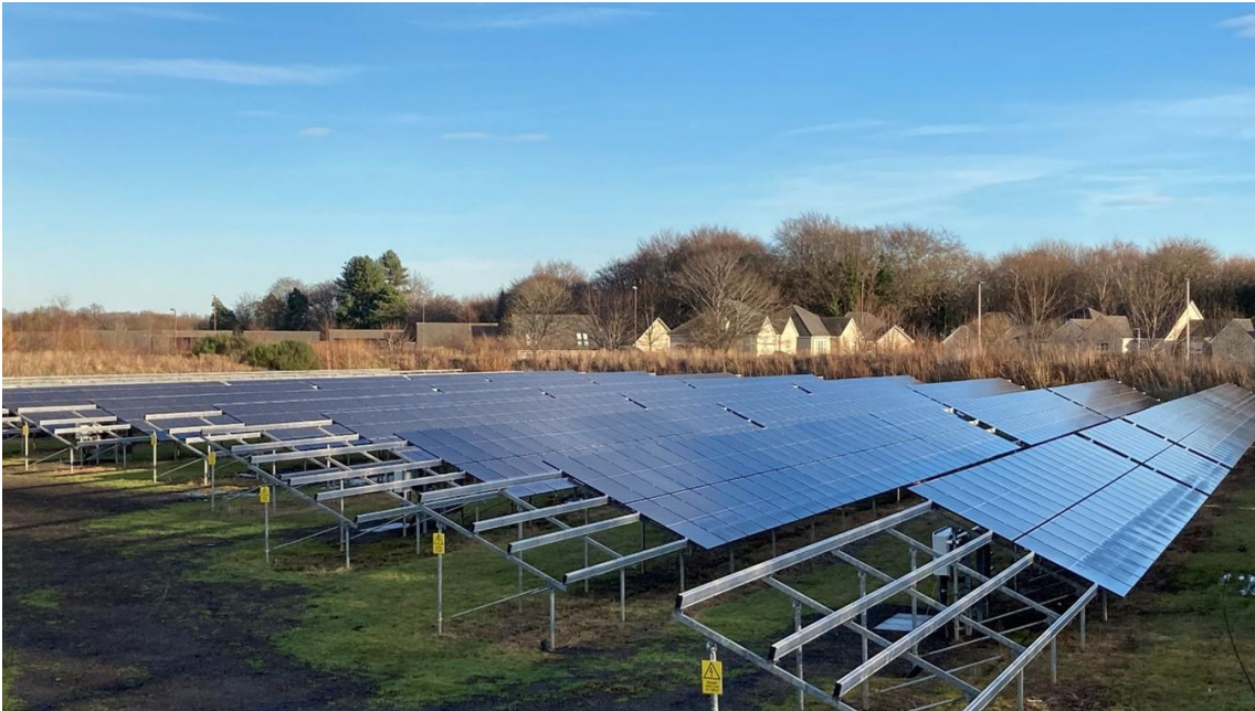
Figure 2.3: Solar panels at Eskbank (Midlothian Council)
